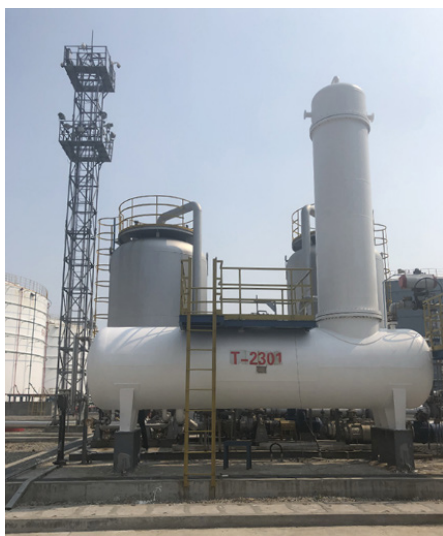
(c) 某油气预处理吸收塔罐
