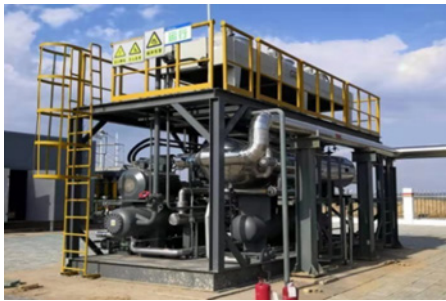
(c) 某油田天然气冷却 (风冷)
