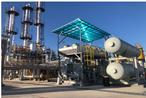
图7.2-1 辽宁某油田轻烃回收(R290/R170复叠-68℃蒸发)
